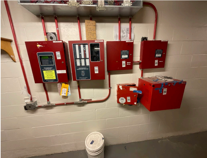
31 - FIRE ALARM SYSTEM
