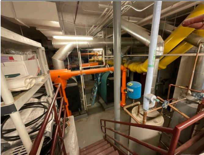
19 - MAIN BOILER ROOM
